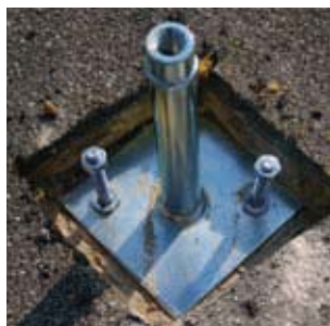
Ritaglio dello strato composto da guaina + isolante e fissaggio piedino Scrap of coating composed by sheath + insulator and fixing foot
